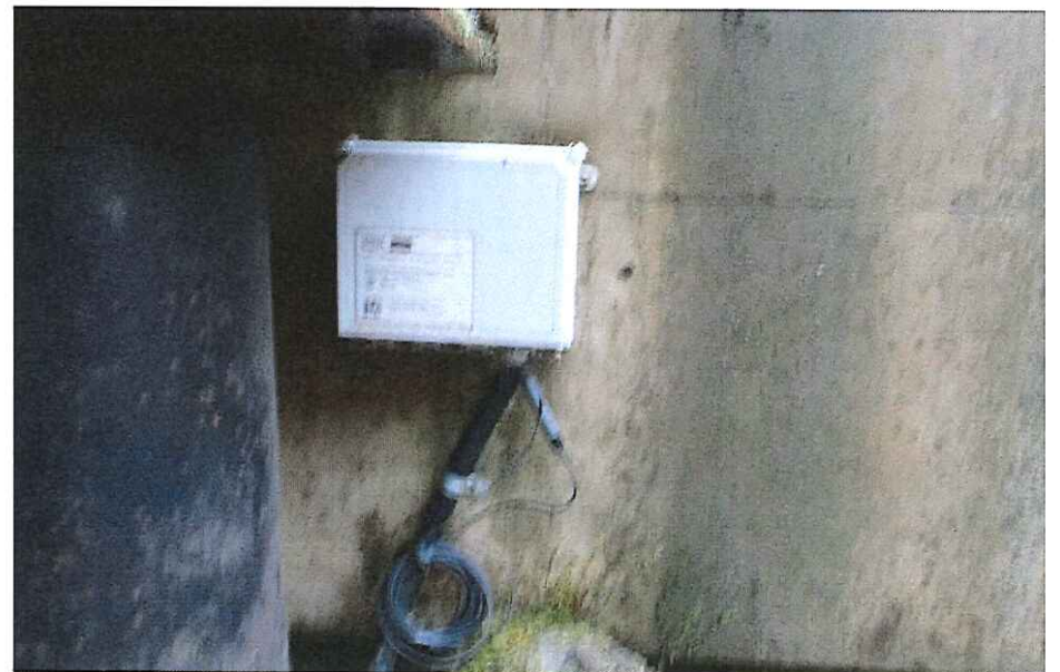
CK2067 data logger
