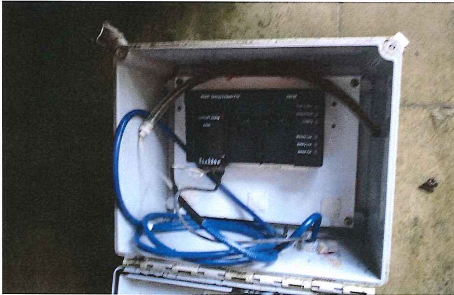
CK2067 data logger 2
